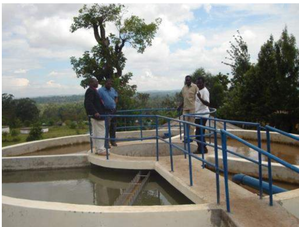
Figure 6: A new clarifier constructed with funding from the SMM project at Angurai Water Treatment Plant in Western Kenya.
